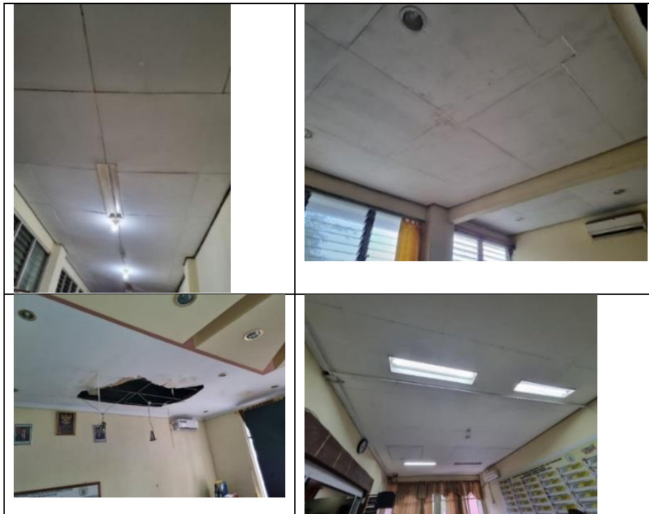
Figure 8 Damage of Ceiling
