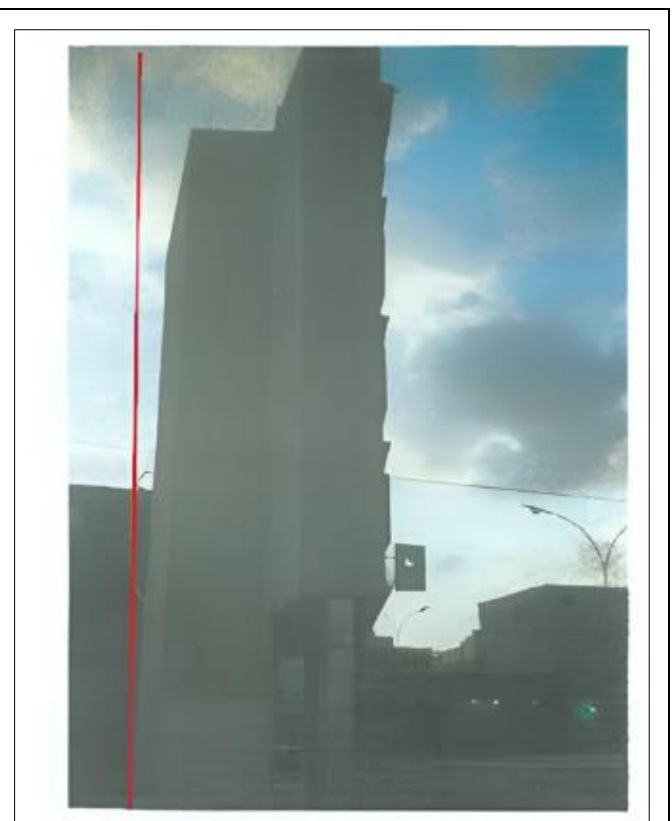
Figure 3 General view of the building after tilt
