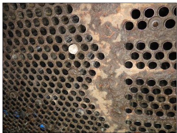
Figure 3 Plugged tubesheet face
